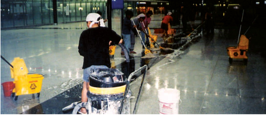
No Skidding® Anti-Slip Treatment was used on the new Hong Kong International Airport, the largest ever application of an anti-slip treatment. This terminal is designed to receive 85 million passengers annually. No Skidding® Anti-Slip Treatment was selected because of its effectiveness, ease of application, low maintenance and durability.
